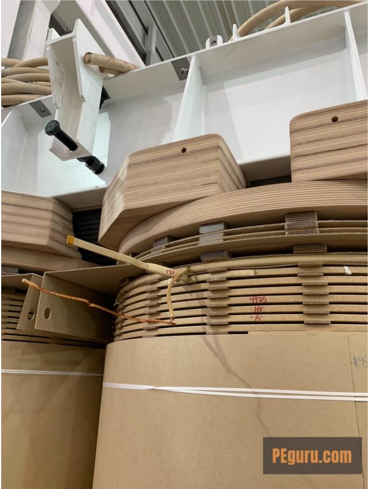
Top clamps that holds the windings in place
