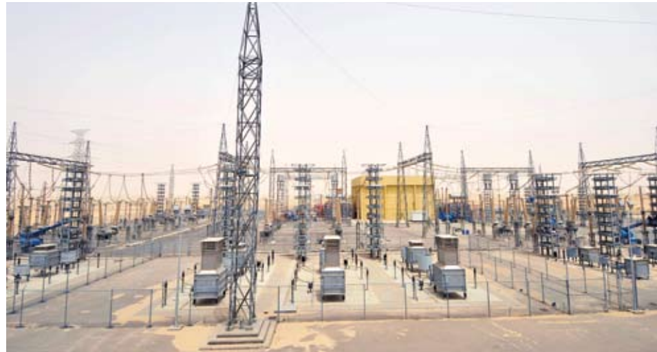
Al Fadhili, Saudi Arabia GCCIA HVDC interconnection
