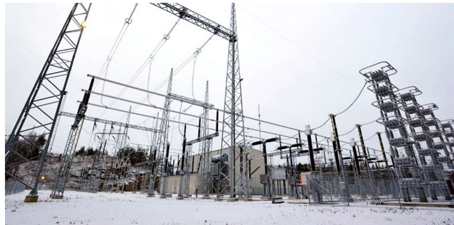
Lindome Sweden : converter substation part of the Konti-Skan HVDC interconnection between Denmark and Sweden
